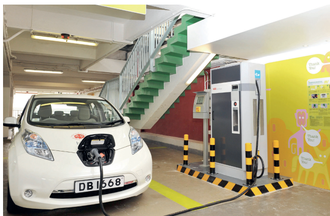
位於天星政府停車場內的電動汽車充電設施 Electric vehicle charging facility at Star Ferry Government car park
